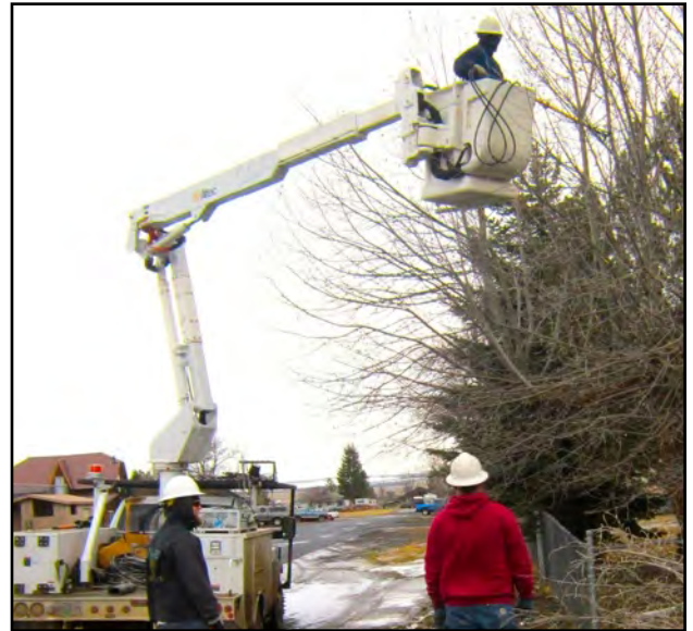
The Columba Power Co-op crew trims trees in Ukiah. The co-op wants to keep the lines clear for 15 feet on each side for safety to prevent power losses during storms.
